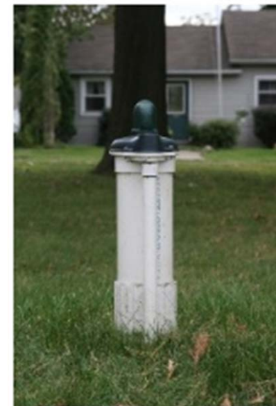
Water Supply Well
