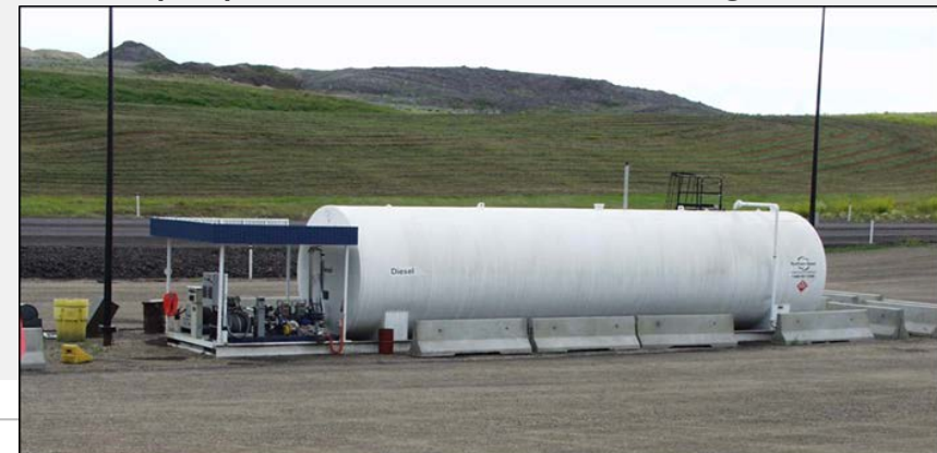
Fuel, propane and lubricant storage facilities
