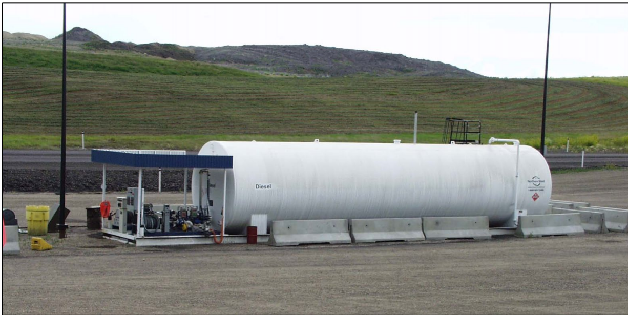
Figure 1.18-1: Example of Pit Fueling Station
