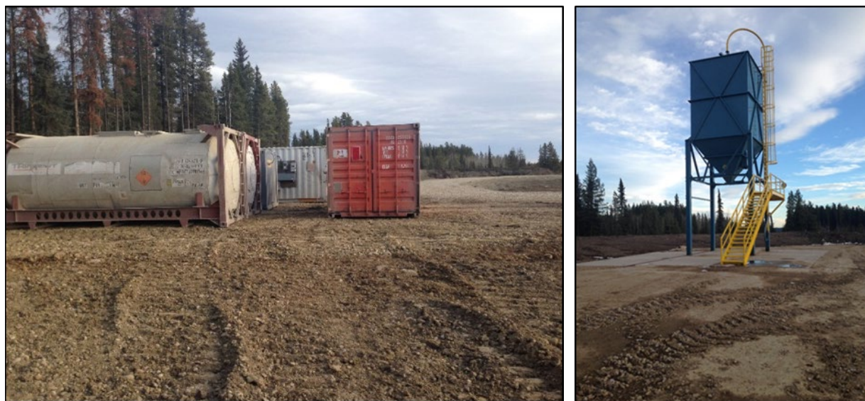
Figure 1.18-7: One (1) 30 tonne emulsion silos and one (1) 50 tonne Ammonium Nitrate Fuel Oil (ANFO) silo for Storage
