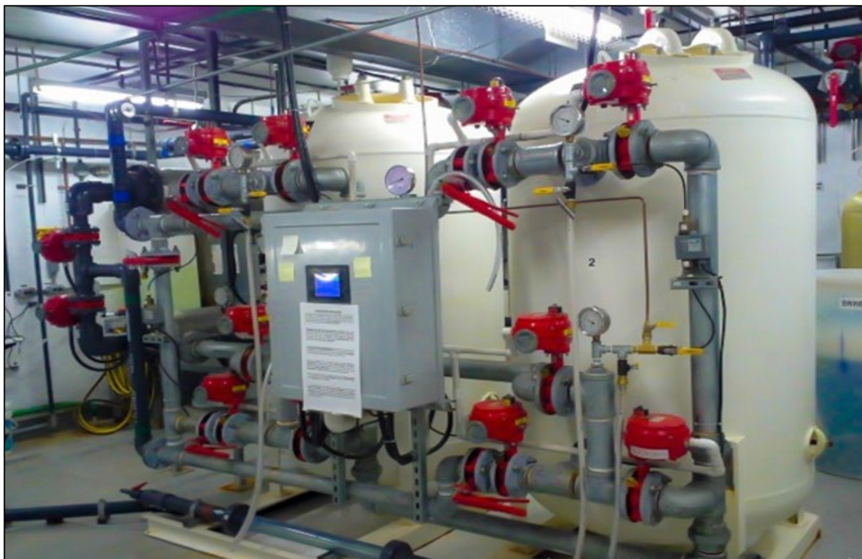
Figure 1.17-4: Example of Potable Water Treatment Plant
