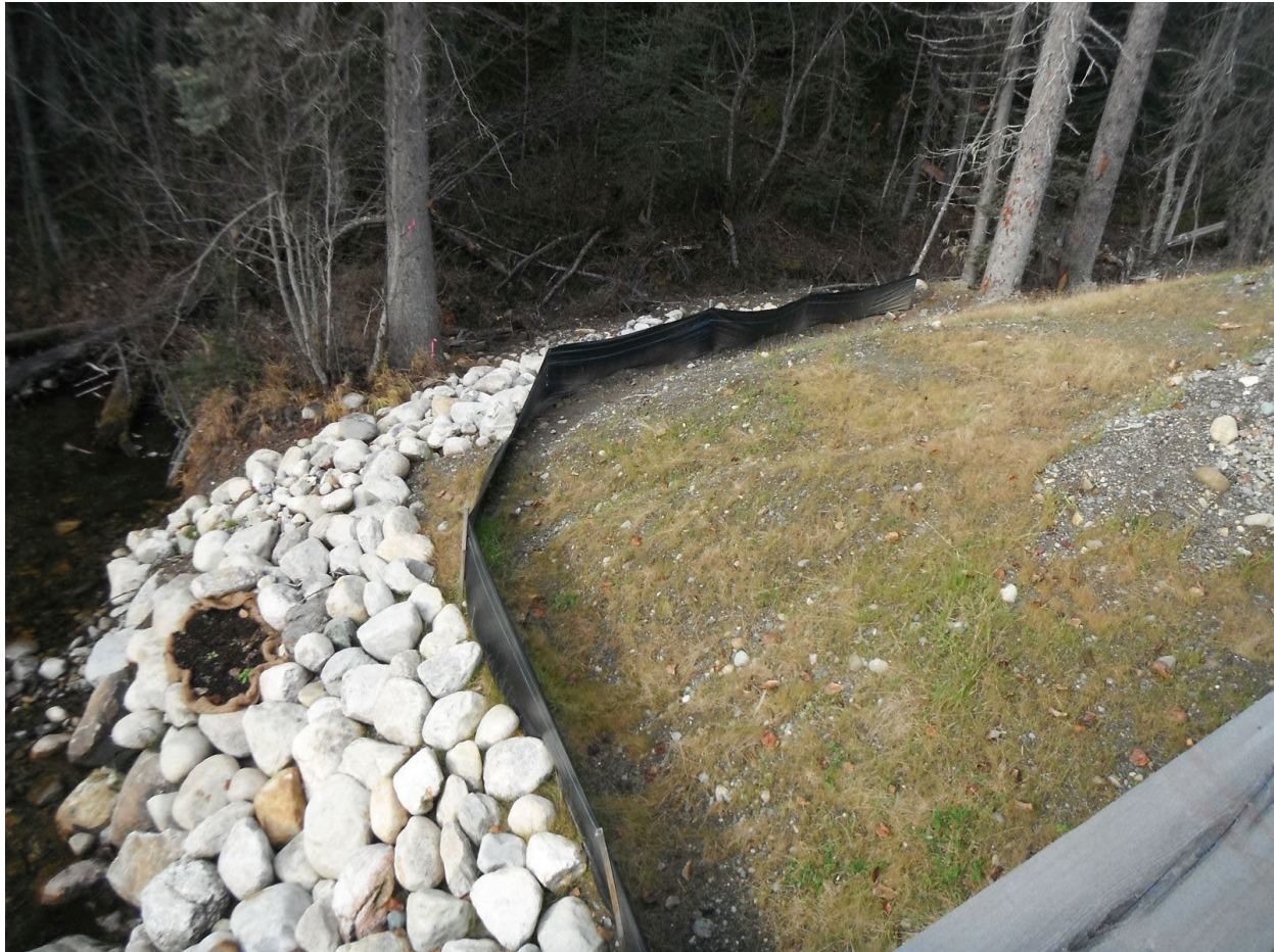
Figure 6.6-2: Example of a silt fence used for sediment control at a bridge site
