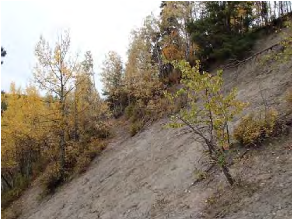
Photo 9: Clayey/silty soils in the landslide initiation zone.
