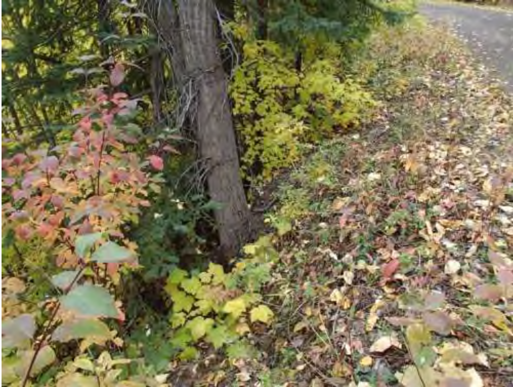
Photo 1: Over-steepened fillslope supported by tree roots and trunks near Sta. 11+600.
