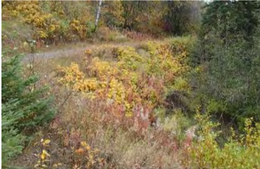
Photo 7: Over-steepened slope below road.
