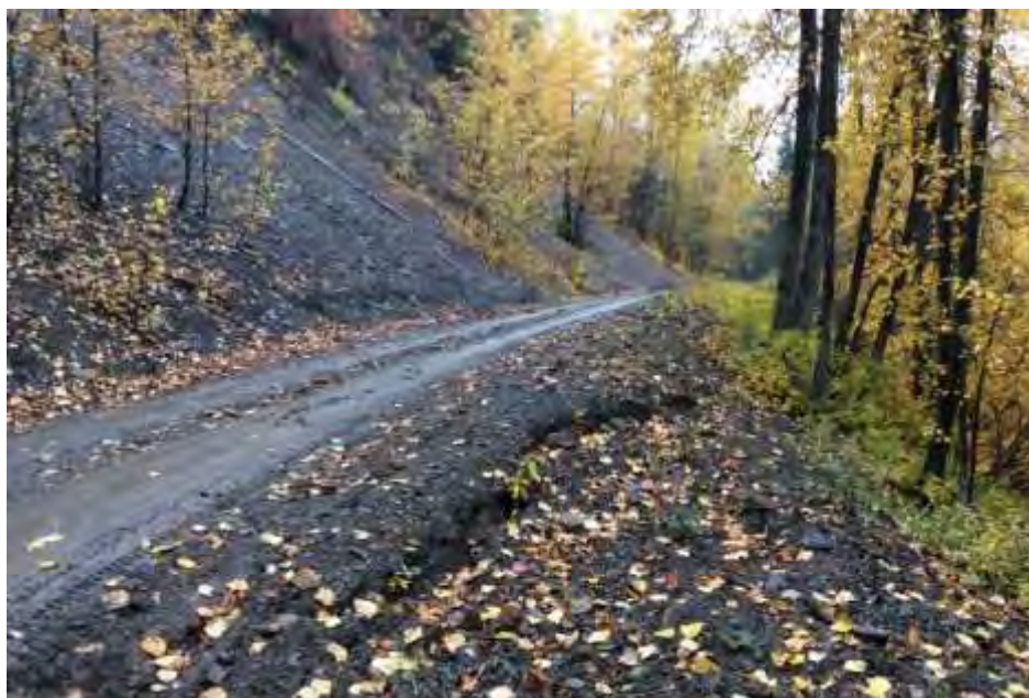
Photo 13: Tension crack in shoulder.
