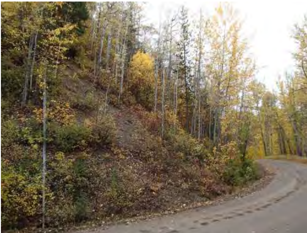
Photo 2: Cutslope at the bend in the road between Sta. 11+640 and 11+700.
