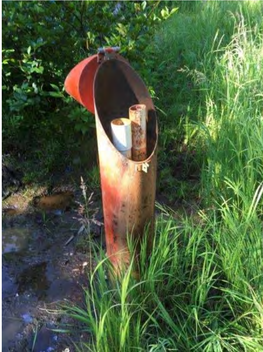
Photo 3 – Well nest T96R-34-67 and T96R-34-67-87. Wells are in good shape although the caps are missing.
