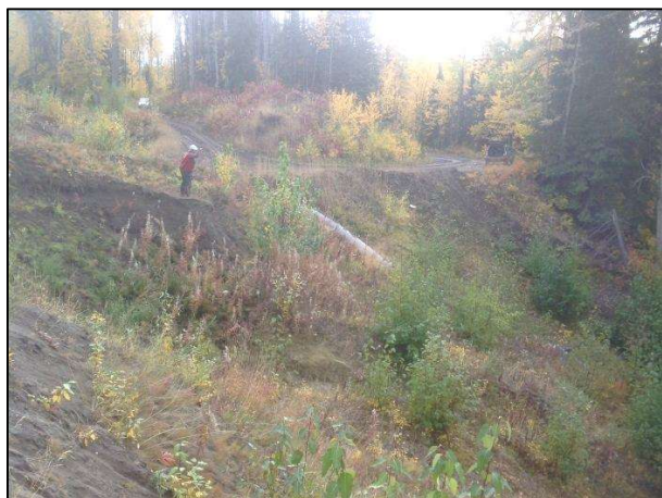
Plate 2-26: Start zone of the Coalmine Road landslide; field sites IW065, IW235.
