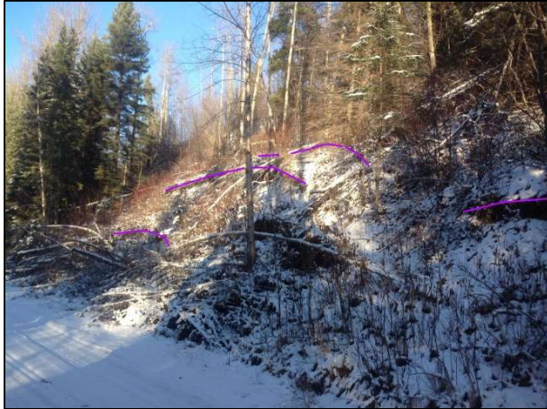
Plate 2-28: Soil creep and tension cracks (purple mark-up) on the steep slope above Coalmine Road; field site IW064.
