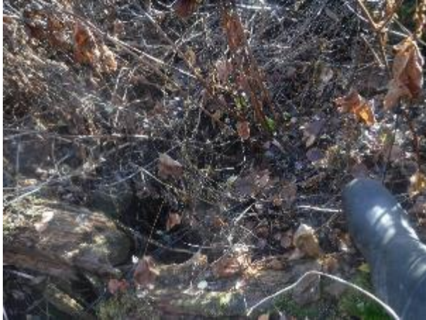
Photo 61: Scoured bowl but organic/discontinuous above the drop.
