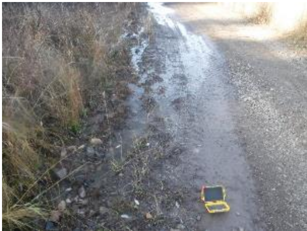
Photo 51: Overland flow onto powerline road (~50 m downslope from crossing).
