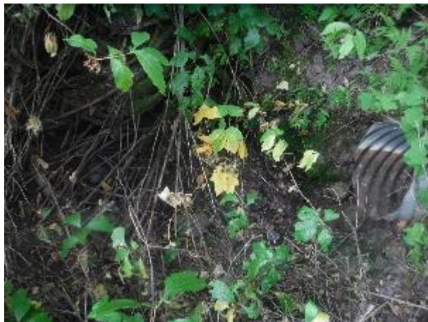
Photo 31. Downstream view of 450 mm culvert with 0.70 m perch.
