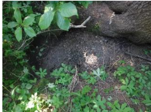
Photo 12. Small section of scour and alluvium (< 1m).
