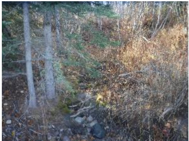
Photo 60: Upslope approximately 10 m from the crossing. Discontinuous section of scour.
