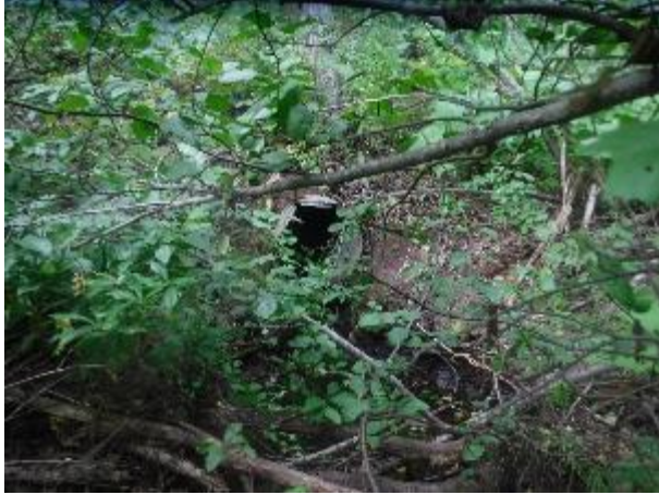
Photo 23. Outlet of 900 mm culvert showing perched outlet.
