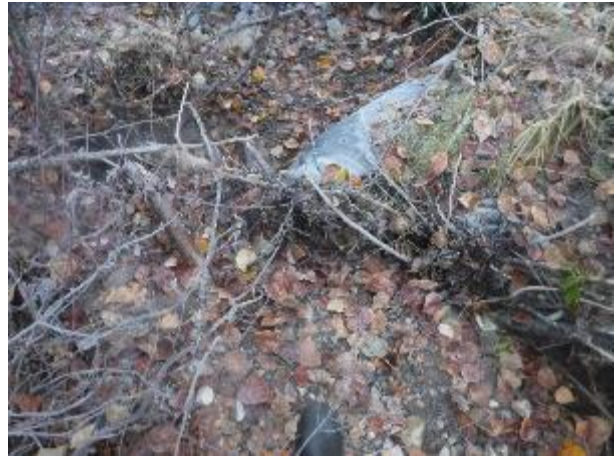
Photo 73: Two plugged 600 mm culverts at the crossing.
