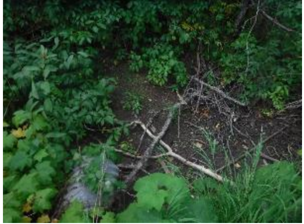
Photo 36. Upstream view of 500 mm culvert. Abundant fines.
