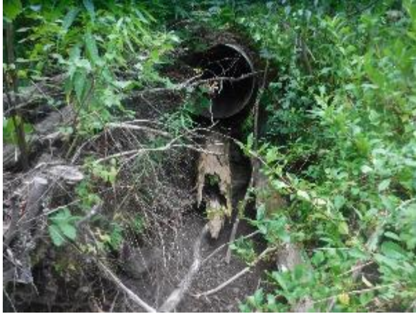
Photo 27. Downstream view of 900 mm culvert with 0.60 m perch at powerline access crossing.
