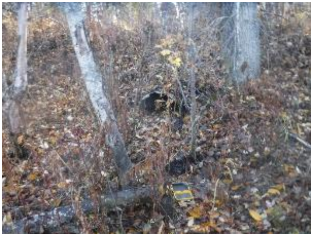
Photo 68: Facing upslope from below road. Culvert is half clogged. Fill over culvert is roughly 1 m.
