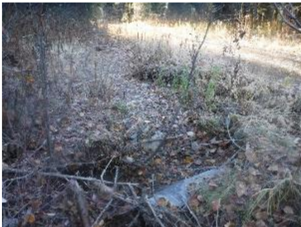
Photo 74: Poorly oriented culverts have been clogged by erosion, directing water down ditch.
