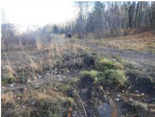
Photo 47: Built BC Hydro road along access corridor is being eroded by excessive braiding.
