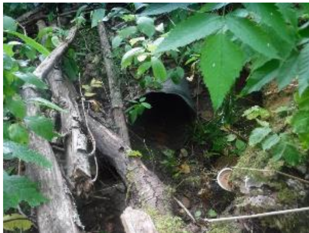
Photo 32. Upstream view of 450 mm culvert. Abundant SWD.
