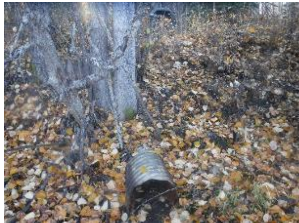
Photo 65: Dilapidated 500 mm culvert below the road. Approximately 1.5 m fill.
