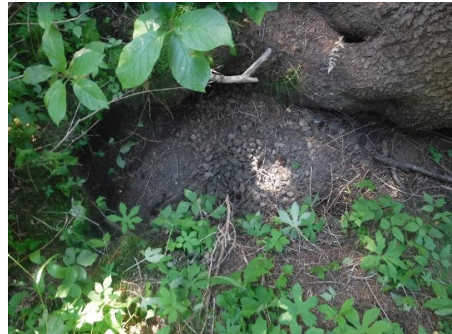
Photo 12. Small section of scour and alluvium (< 1m).
