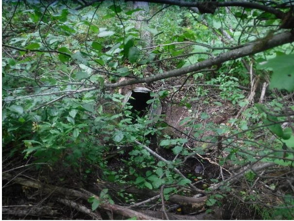
Photo 23. Outlet of 900 mm culvert showing perched outlet.
