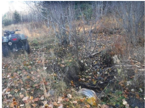
Photo 48: The 600 mm CMP on the BC Hydro road is too small and erosion occurs during peak flow.
