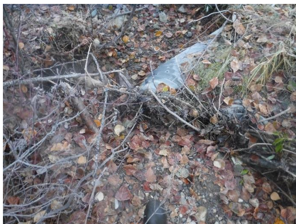
Photo 74: Two plugged 600 mm culverts at the crossing.
