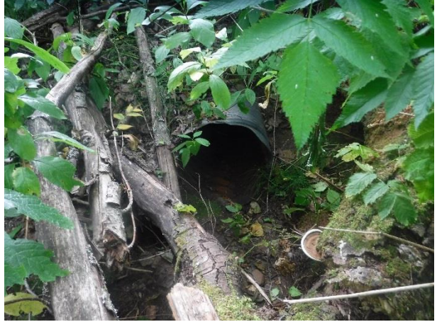
Photo 32. Upstream view of 450 mm culvert. Abundant SWD.
