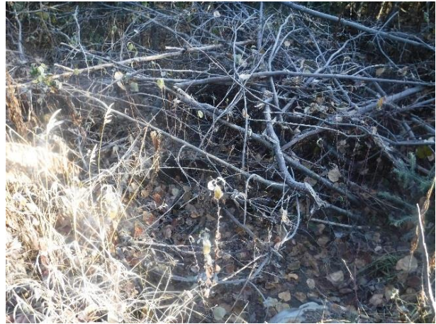
Photo 76: Downstream side of crossing. Some water still uses this old channel.
