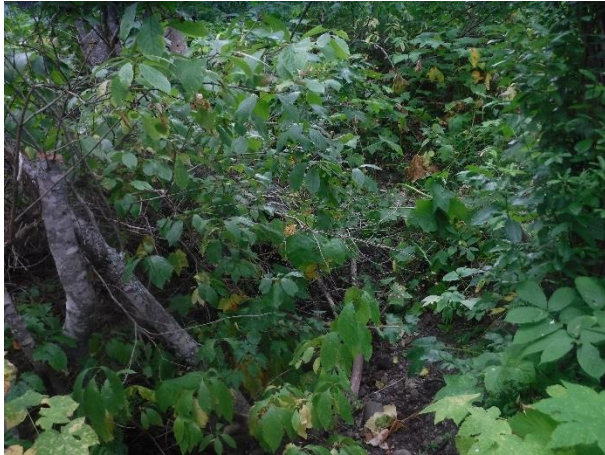
Photo 35. Abundant overhanging vegetation obscuring the 500 mm culvert present at the crossing. Downstream view.
