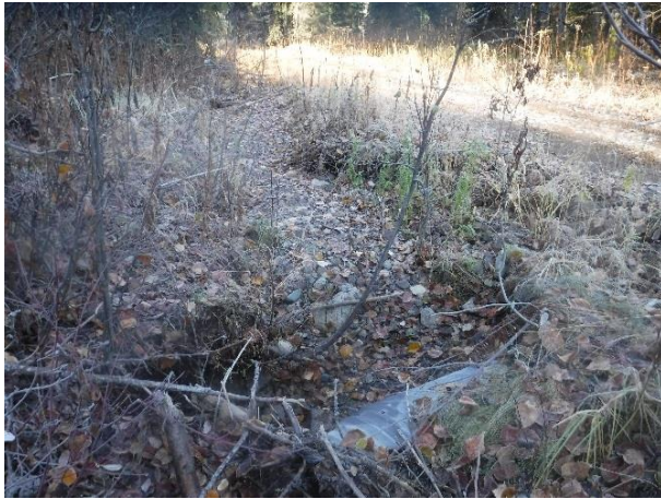
Photo 75: Poorly oriented culverts have been clogged by erosion, directing water down ditch.
