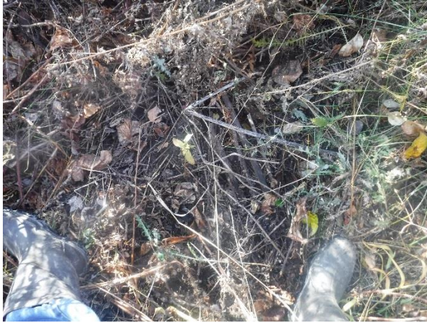
Photo 57: Lack of channel/scour located approximately 50 m downslope of crossing.
