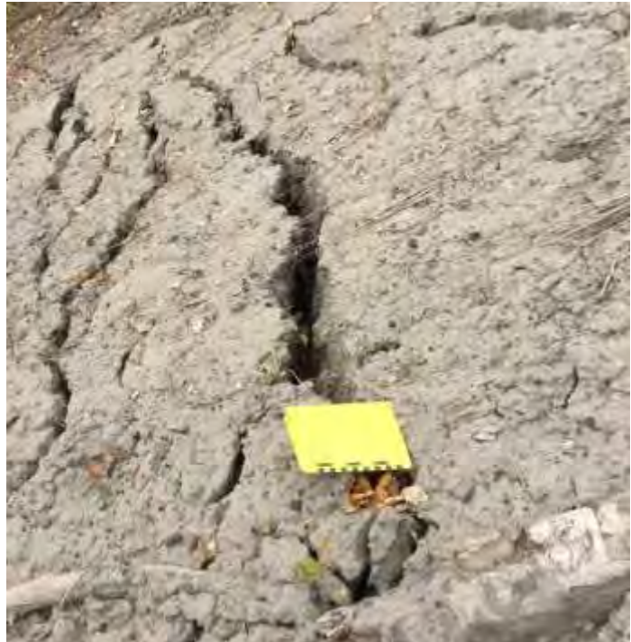
Photo 10: Open cracks in the landslide surface.
