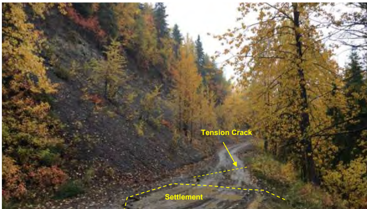
Photo 12: Settlement and tension cracks near Sta. 13+920 to 13+930.
