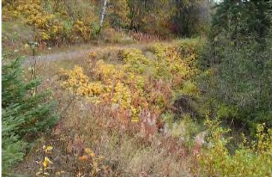
Photo 7: Over-steepened slope below road.
