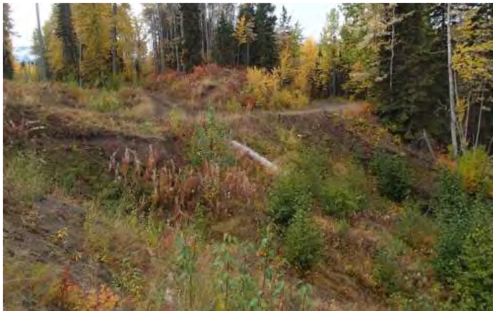
Photo 1: Overview of fillslope failure with the culvert in the middle of the photo and the other bowl to the left. Note the junction with Caribou FSR01. Goathorn Creek Road continues to the right.
